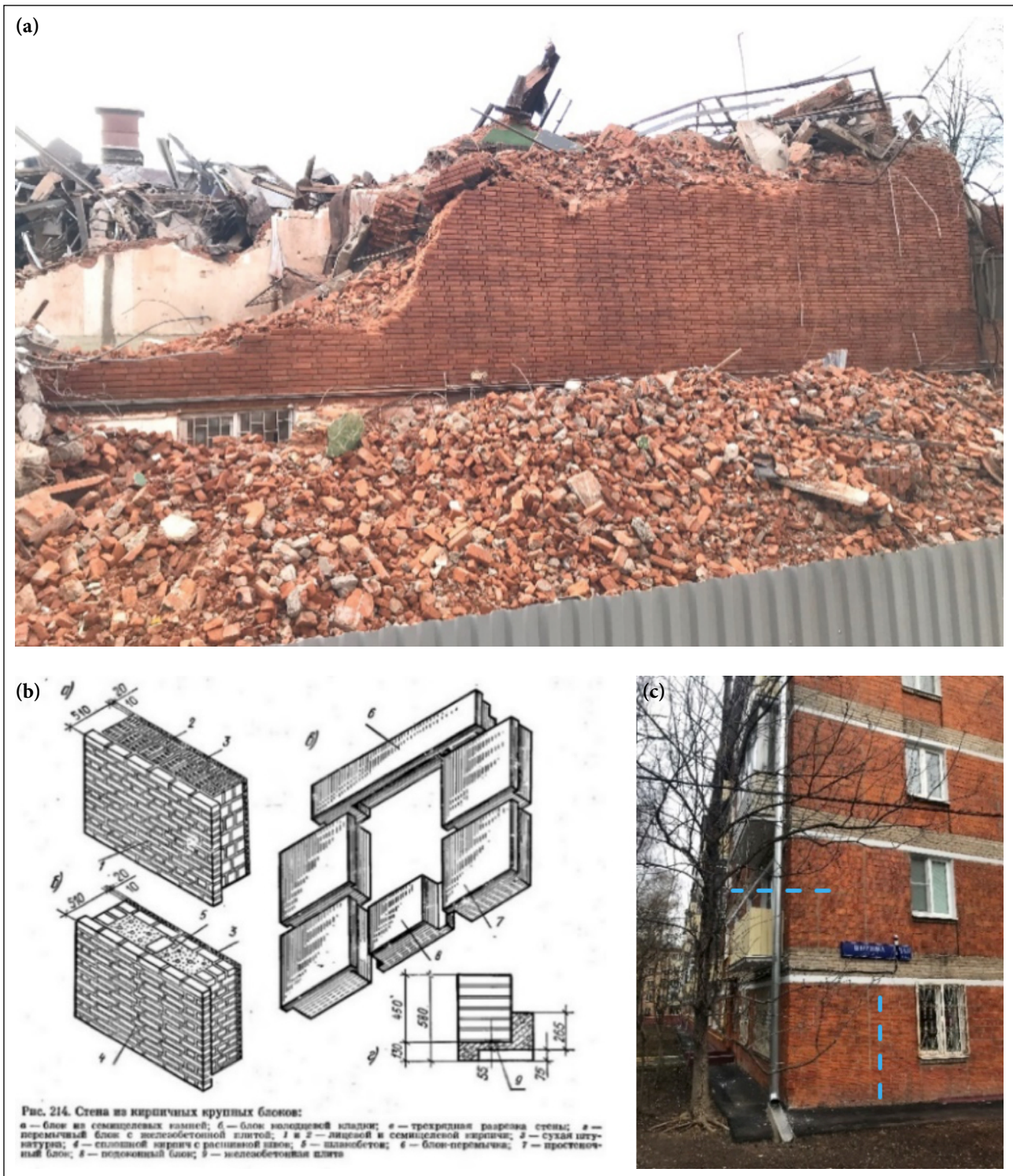
Figure 5. (a) The Vityaz Movie Theatre's brick walls were captured during demolition. (b) Schematic drawing illustrating construction with pre-built large masonry-block wall panels [38]. (c) The five-story mass housing project was constructed with prefabricated large-block brick wall panels in the 1960s–70s Moscow.
